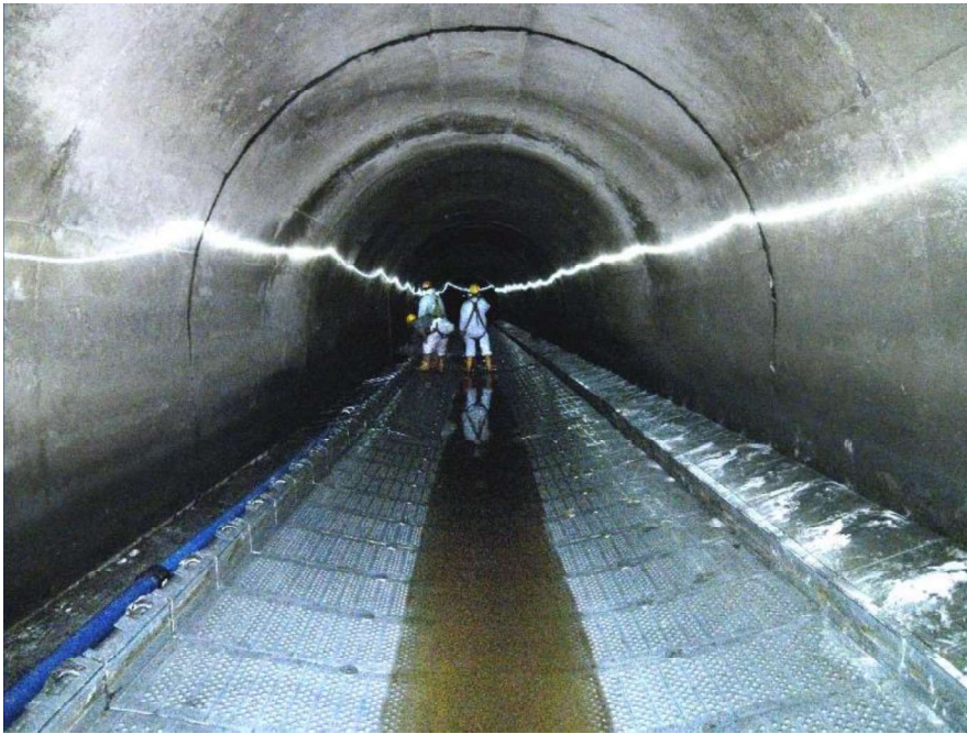
Waste-Water Channel with stainless steel heat exchangers as heat source for the heat pump
